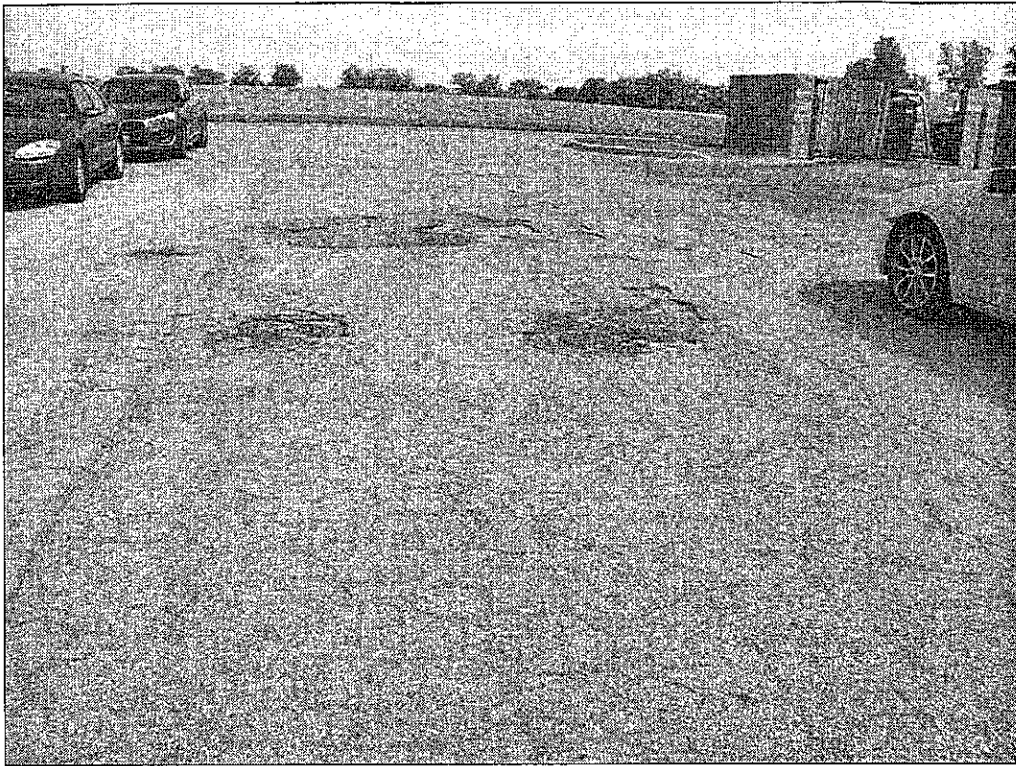
Parcel APN 17-6.0-23-000-000-038.000 – looking north – deterioration of driving surface
