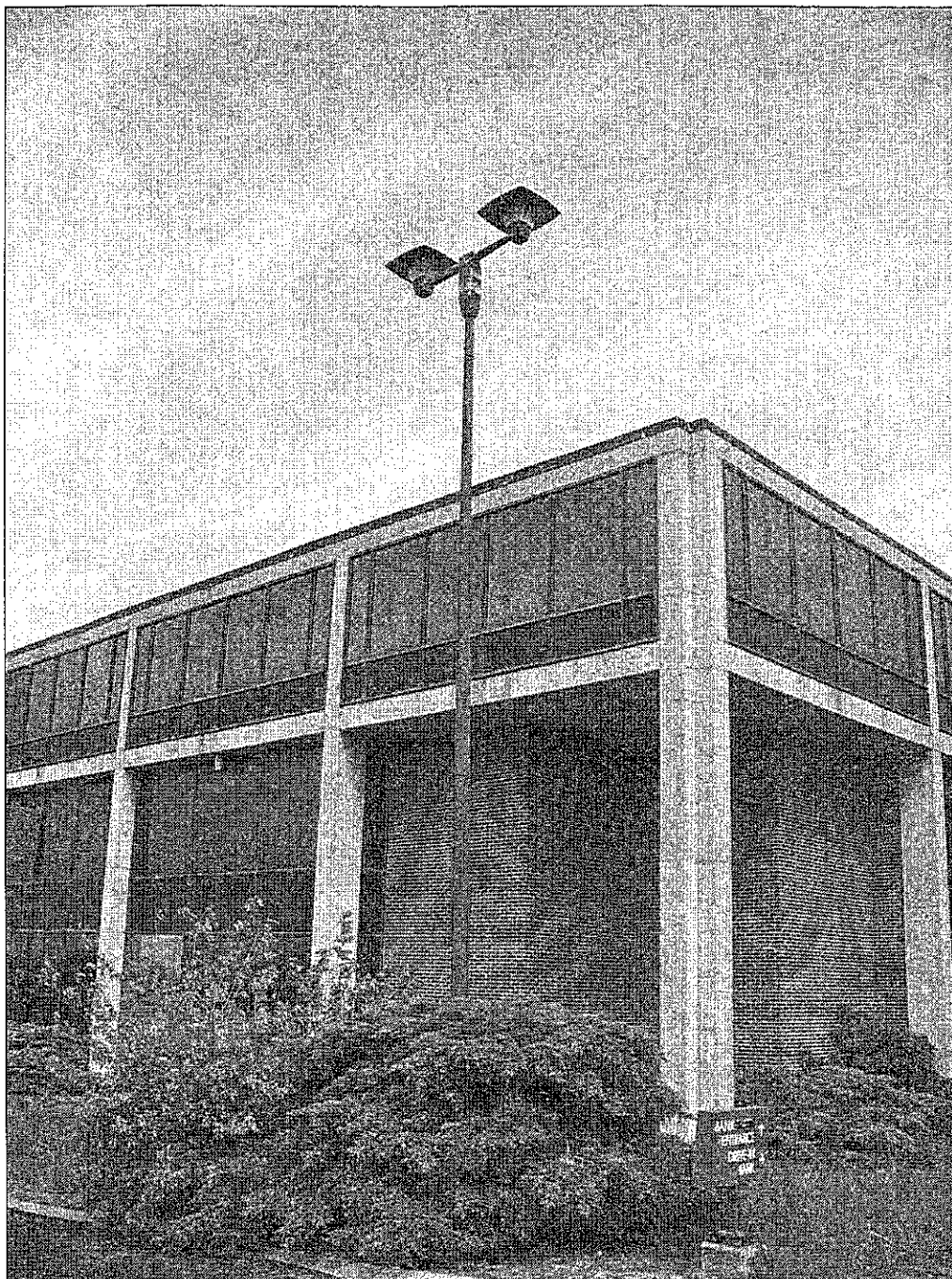
8800 NW 112 th Street – looking northwest – failure of exterior finishes; overgrown vegetation
