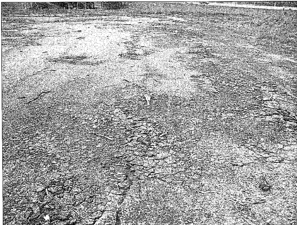
8800 NW 112 th Street – looking southwest – deterioration of parking surface
