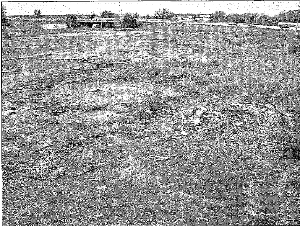
8800 NW 112 th Street – looking southwest – deterioration of parking surface; debris
