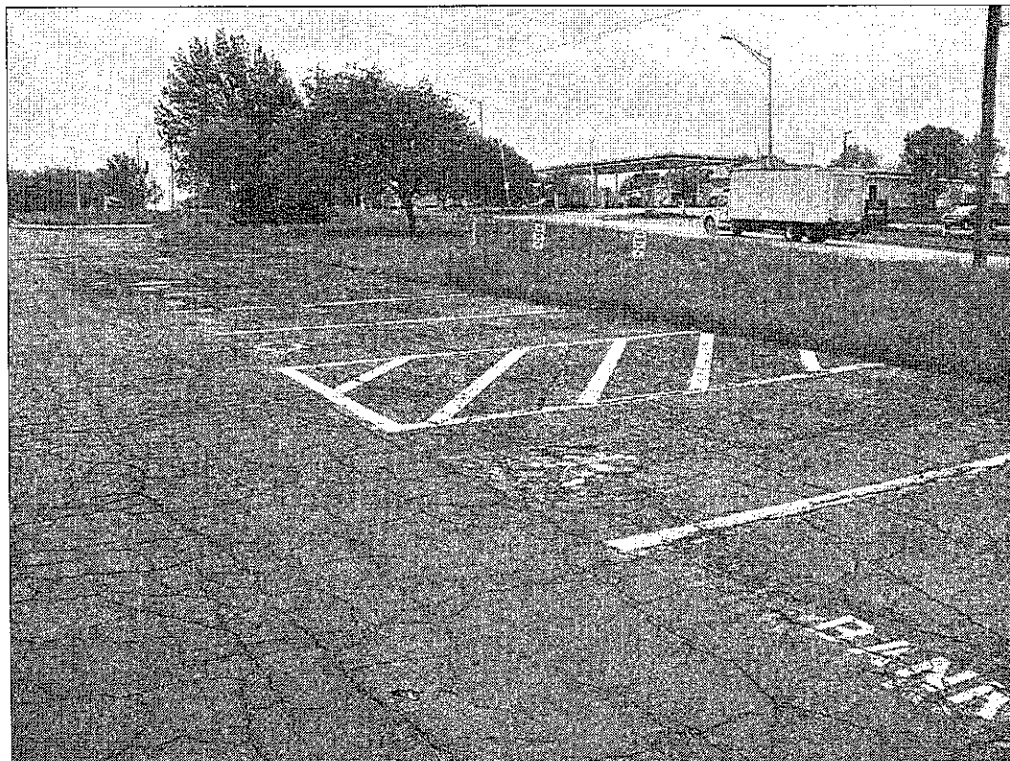
8800 NW 112 th Street – looking southeast – lack of code compliant accessible signage, wheel stops
