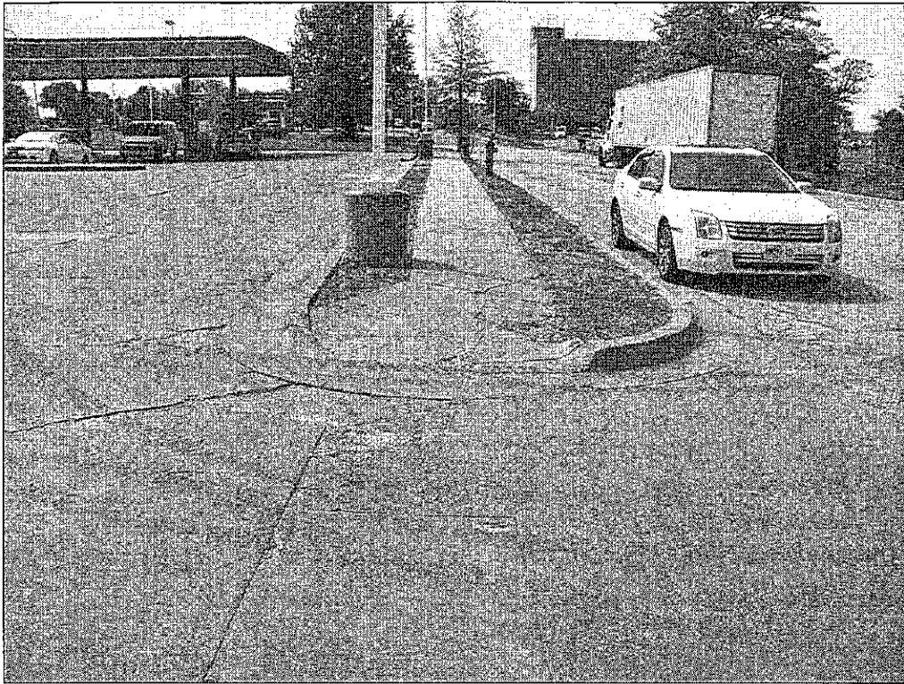
Parcel APN 17-6.0-23-000-000-038.000 – looking south – broken/uneven sidewalk; noncompliance with ADA code
