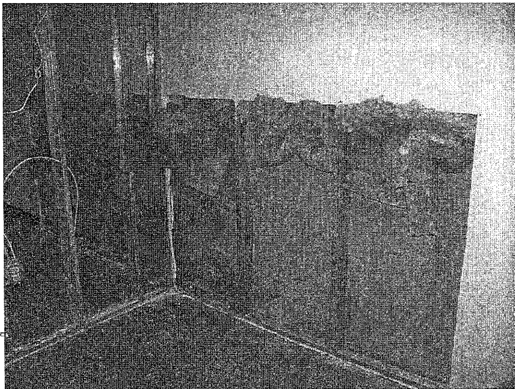
8800 NW 112 th Street – interior of third floor – evidence of water intrusion
