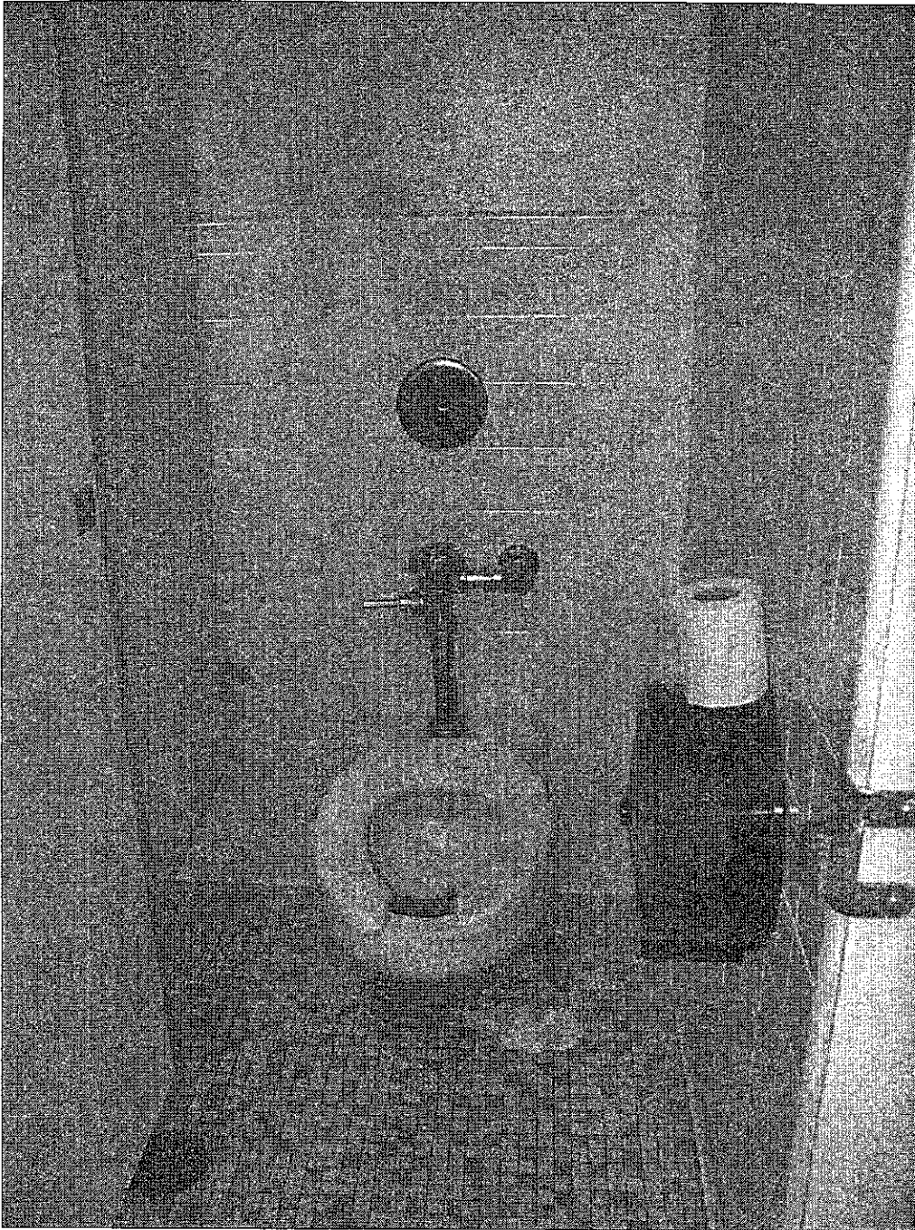
8800 NW 112 th Street – interior – noncompliance with ADA code (single stall restroom)
